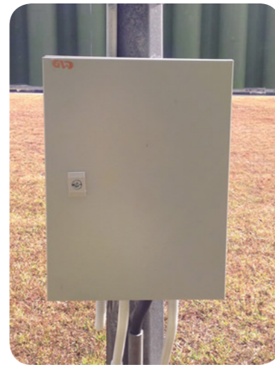
GW enclosures installed at Macritchie Reservoir for camera surveillance system
